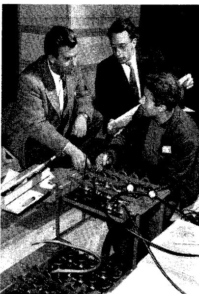
H. Bakker (centre) and J. Thorlund belong to the proton synchrotron Control section which is responsible for the cable layout. Here they discuss the laying of cables with a workman from an outside firm.
